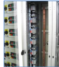
Auxiliary and cable area: located in the cable compartment or in the rear area in the single cabinet.
